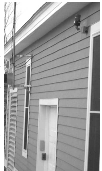
Emergency light located on upper right to the garage door entrance to the Waste Water Treatment.
