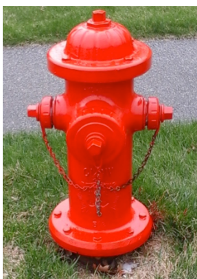
Thanks to Peter Abate and Dom DeFronzo, VSR hydrants received a long overdue facelift (Safety Red) on work play day.
